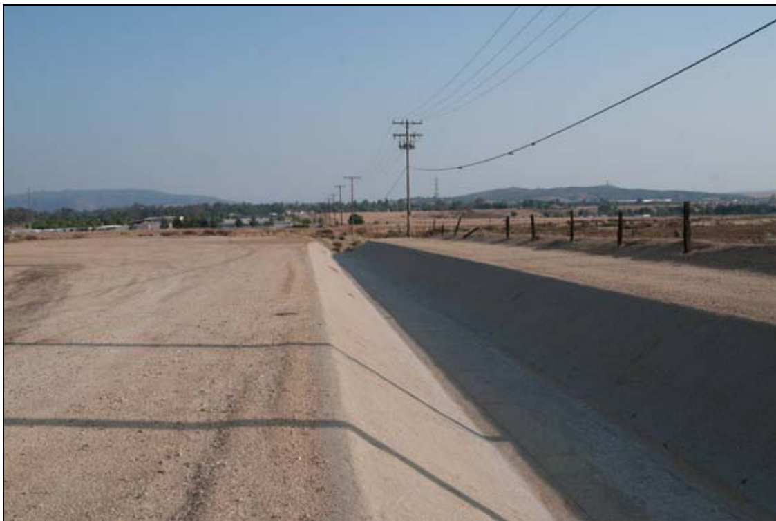
Photograph 4: Looking south showing the concrete section of Mountain View Channel, north of Noble Creek.
